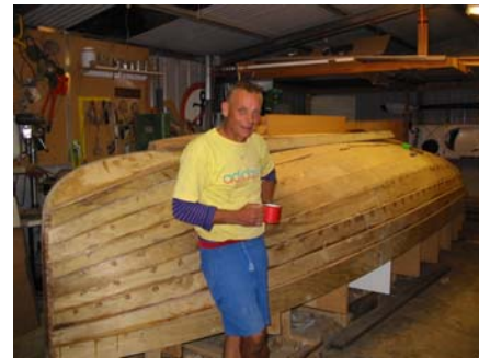
Colin Wragg of Pt Sorell with his new “Snapper Boat” under construction
